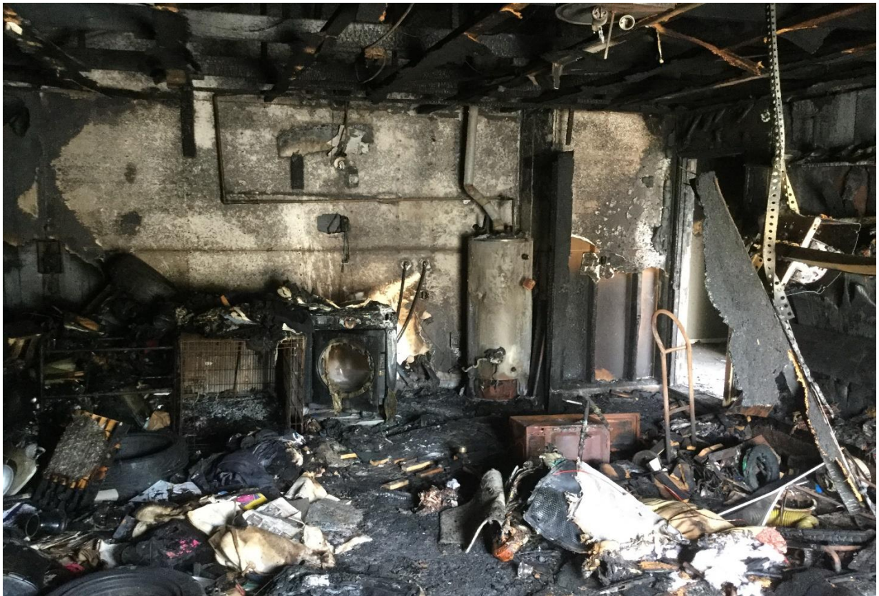
The above photo is an example of a garage that was destroyed by fire. Numerous items and materials here likely contained lead.
